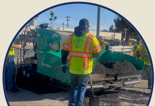
Santa Maria Public Works uses the new state-of-the-art paver funded by Measure A
