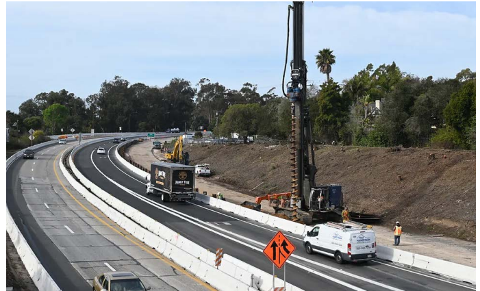
Construction begins on Highway 101 in the City of Santa Barbara between Olive Mill and Hermosillo Roads.
